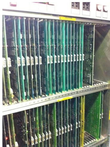
Siemens ISDX Cabinet
